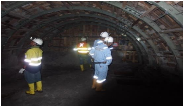
Fig. 11. Steel arch support
